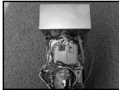
Figure 29: Gas valve assy.
